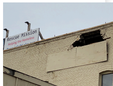
Earthquake damage to the outside of the Rescue Mission. See inside damage on page 3.
