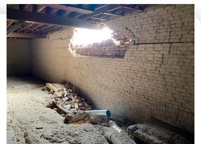
Earthquake damage to the inside of the Rescue Mission. See outside damage on page 4.
